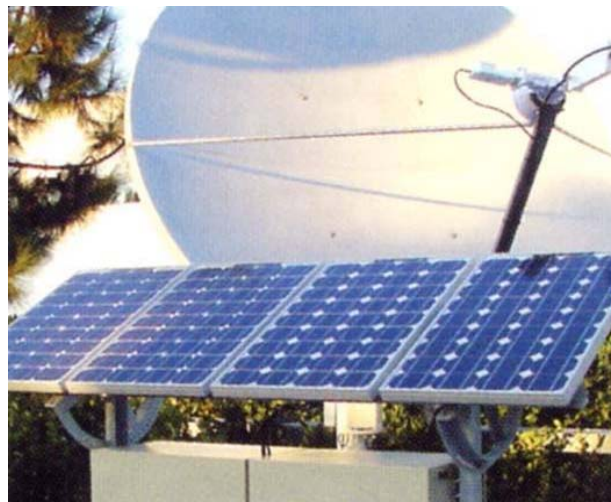
VSAT Equipments powered by Solar
