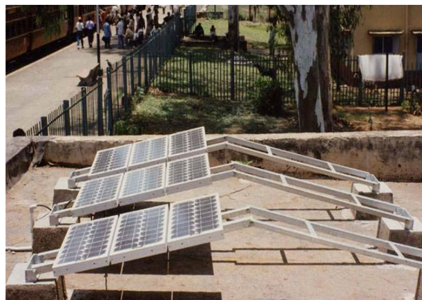
Solar Module at Level Crossing Gates
